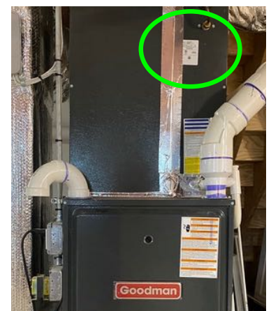
Model number and Serial number location for the cooling coil that is adjacent to the furnace
